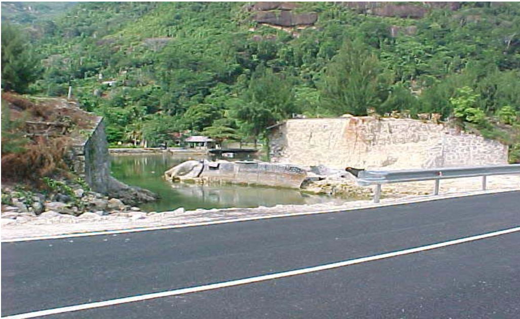
Plate 1: Damaged Cascade Bridge and new diversion road constructed
